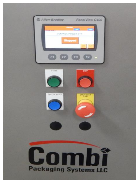
Operator Control Panel
