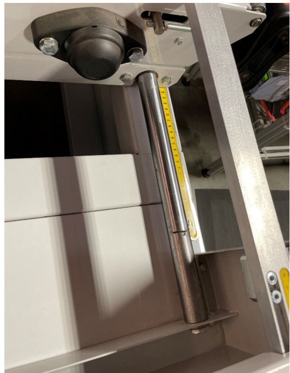
Figure 18. Infeed conveyor linear shaft requiring monthly grease application.
